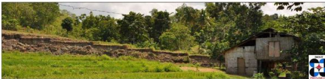
3-meter fault scarp of the North Bohol Fault in Brgy. Anonang, Inabanga
